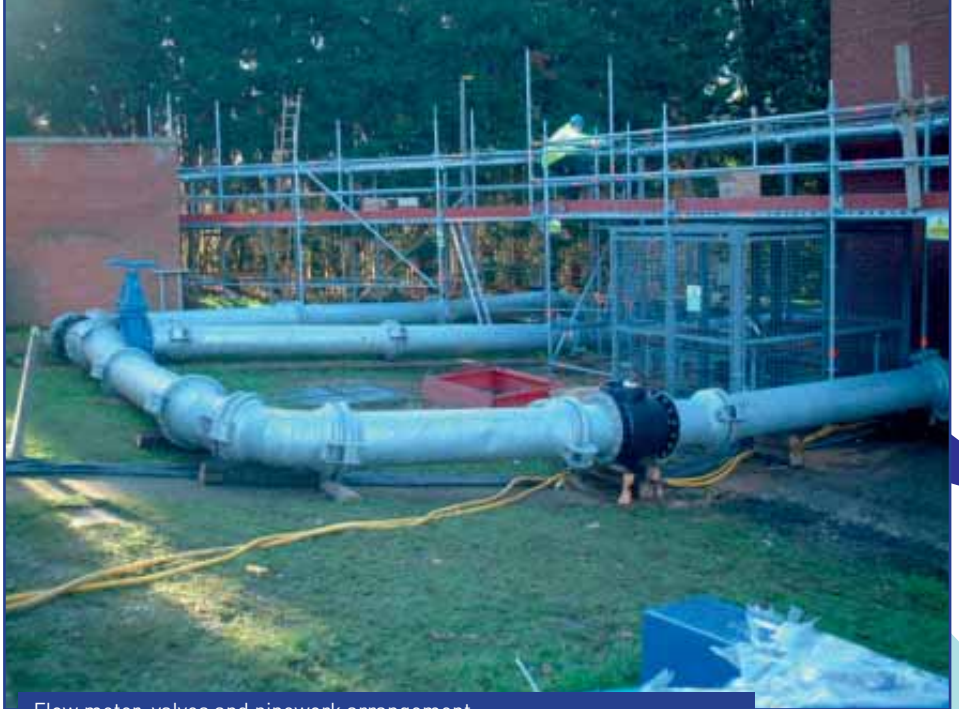
Flow meter, valves and pipework arrangement
