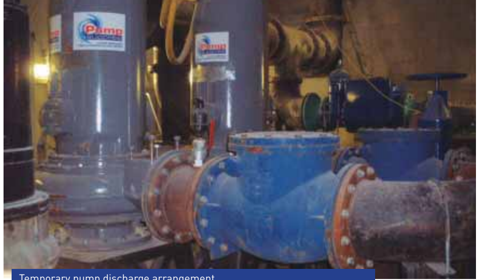
Temporary pump discharge arrangement
