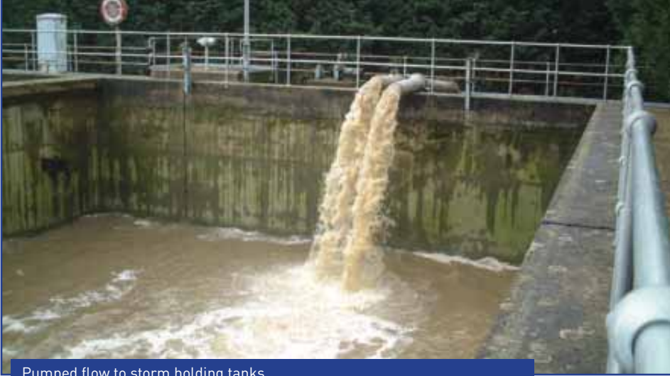
Pumped flow to storm holding tanks
