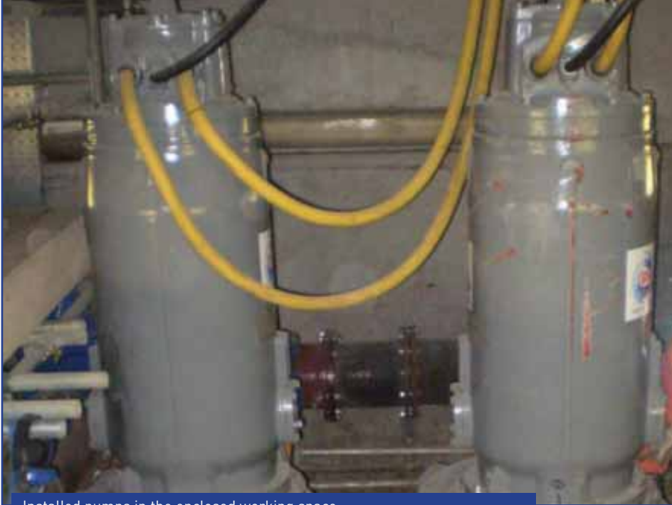
Installed pumps in the enclosed working space
